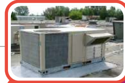
Fully Controlled HVAC System
